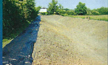
17. The scraped soil is then replaced and work can start on the towpath.
